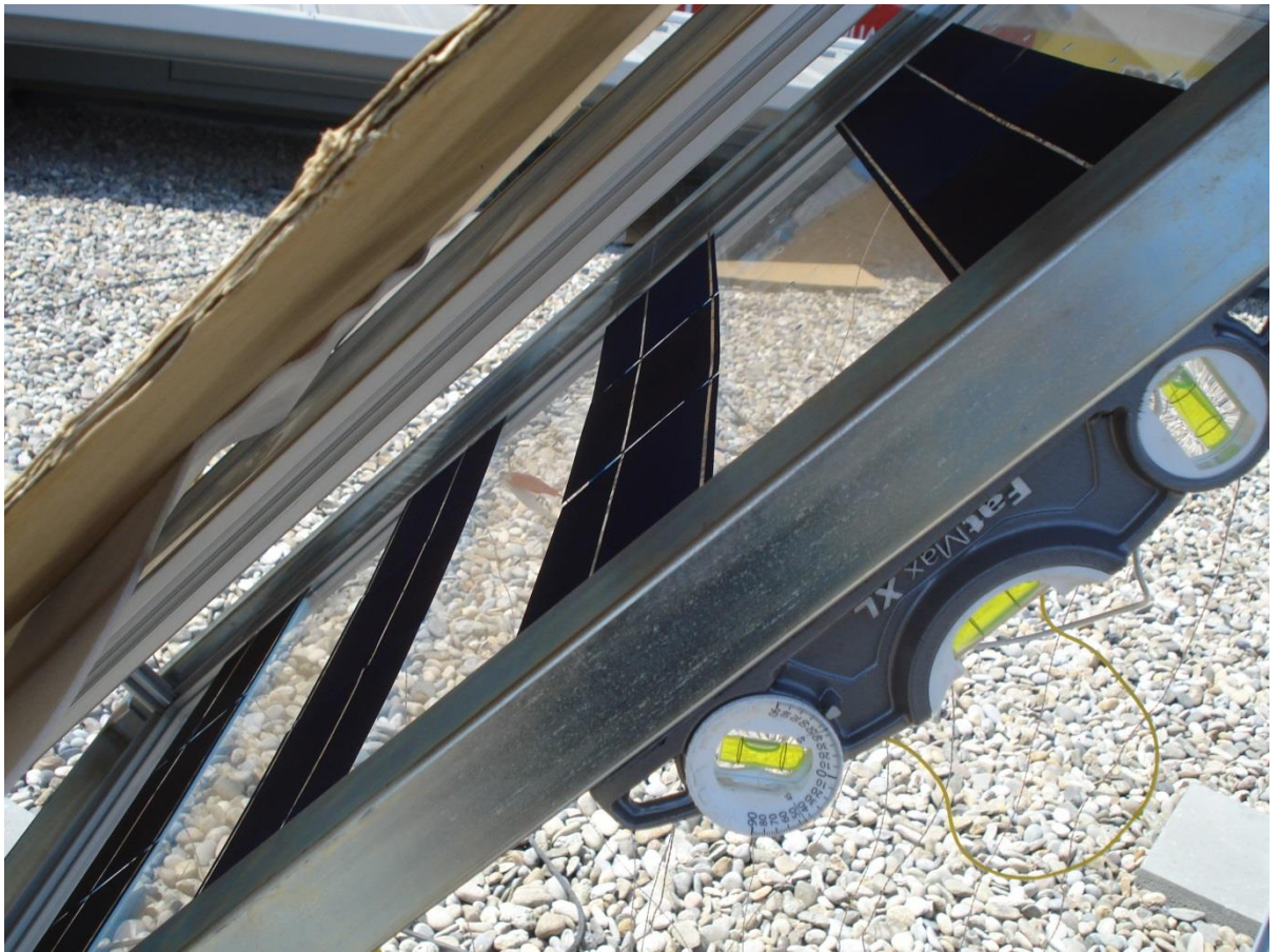
Figure 4-17 – Frame mounted manual inclinometer
