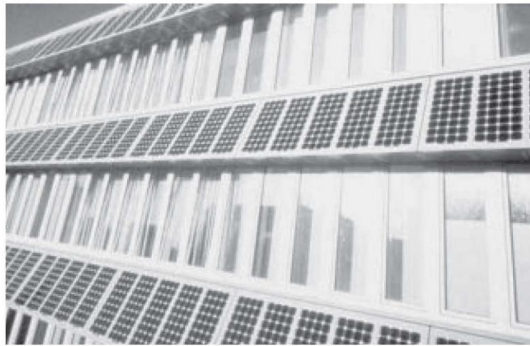
Figure 2-34 – PV modules on an inclined wall
