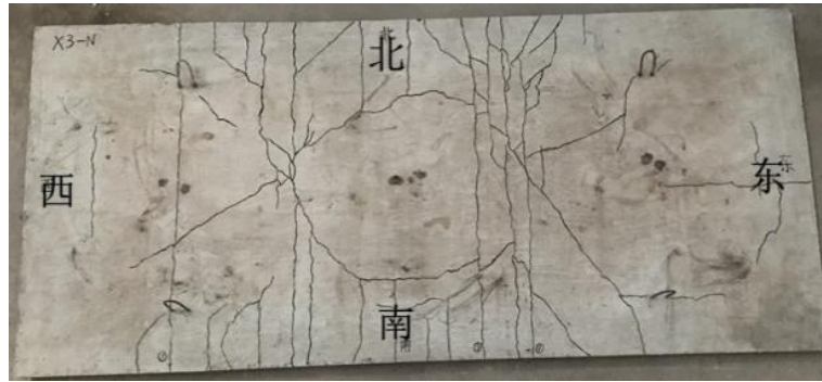
(a) Cracking pattern on the top surface
