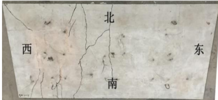
(a) Cracking pattern on the top surface
