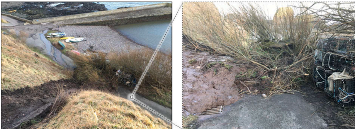
Fig. A.1. Landslide blocking the road down to the harbour from the residences of Catterline following heavy rains in February 2020. Photo credit: Pieter voor de Poorte.
