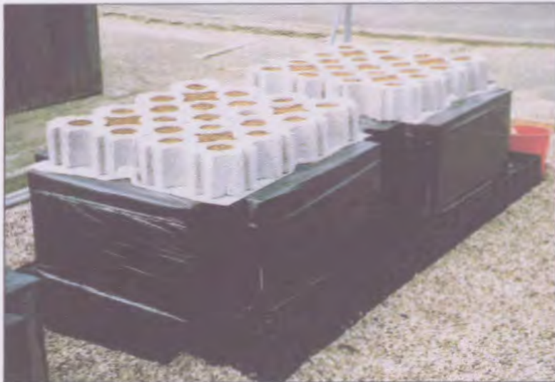
Figure 17 Completion of the rig with growing medium filling the surfacing blocks' voids
