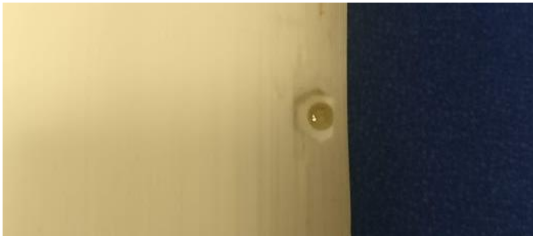
Figure 0.18 Bolt Hole with PVA Blockage
