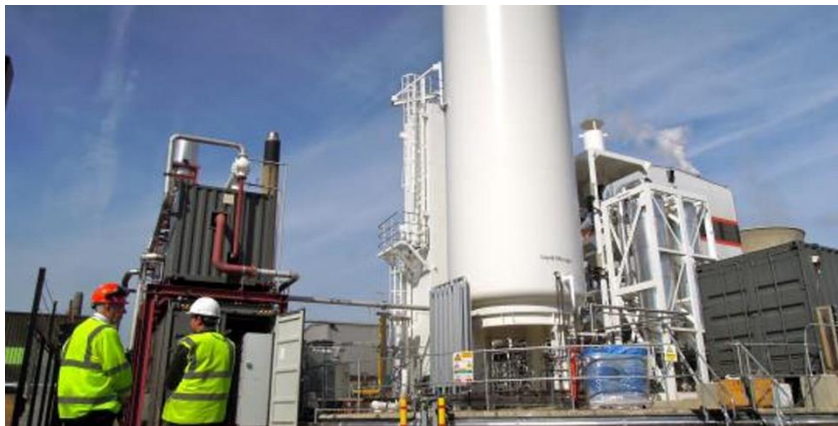
Figure 2.5 – Highview pilot LAES plant, UK 2010 [13]
