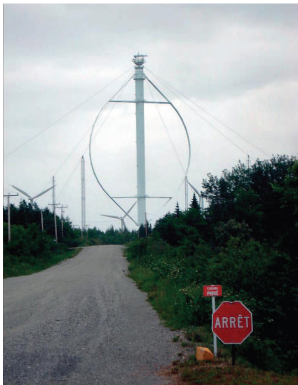
Rycina 18. Turbina Darrieusa w Quebecu, Kanada (fot. Spiritrock4u)
