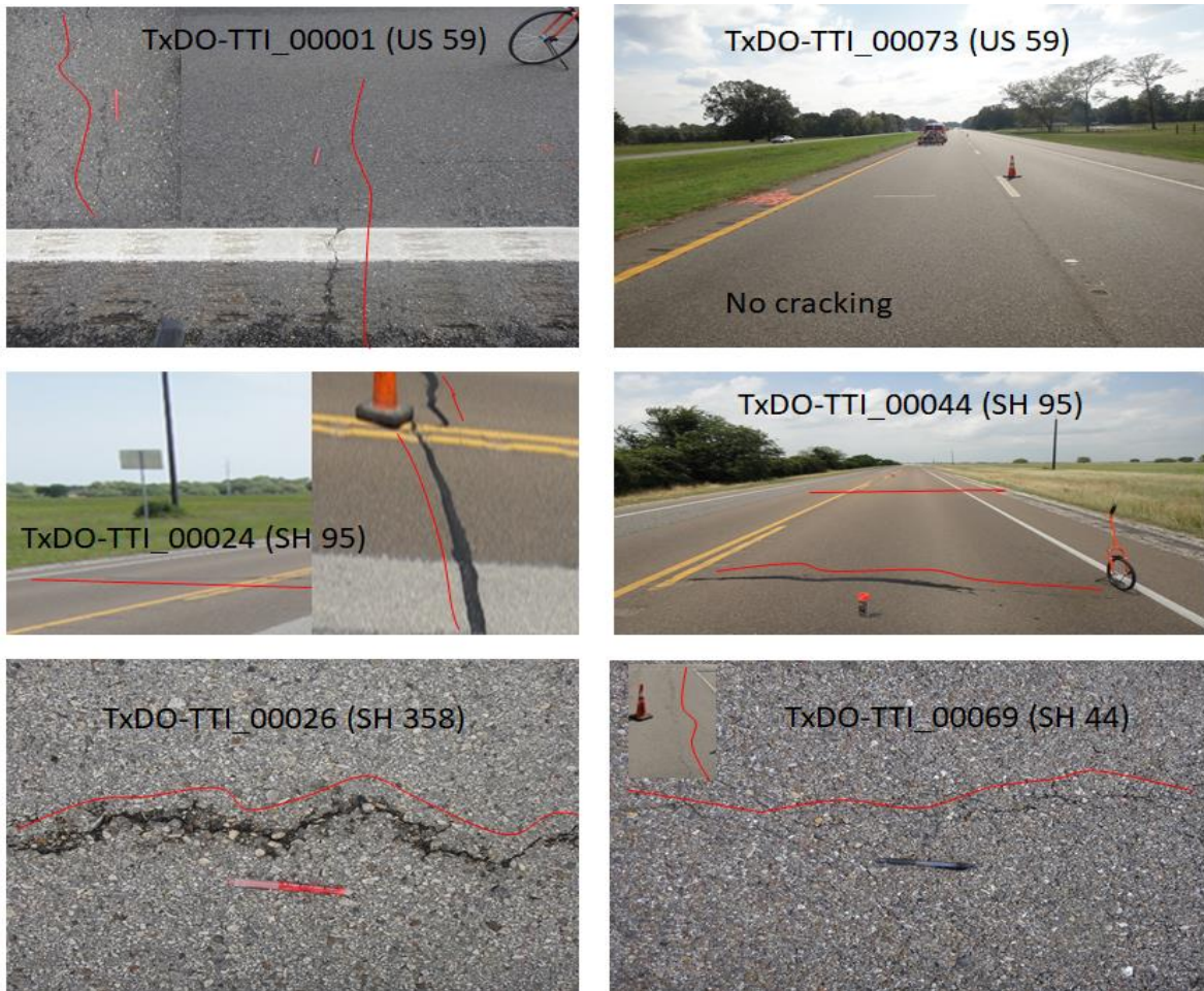
Figure 10. Pavement Surface Condition (Spring 2019).
