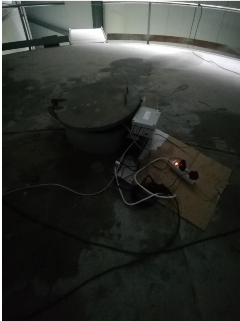
Figure 39 - Assembly on top of the principal tank
