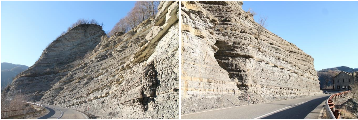
Figures 79. View of Le Scalacce from the ground during the first inspection in January 2020
