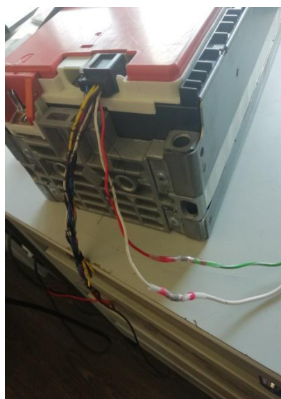
Figure 24 - VW battery module and respective CAN bus connection
