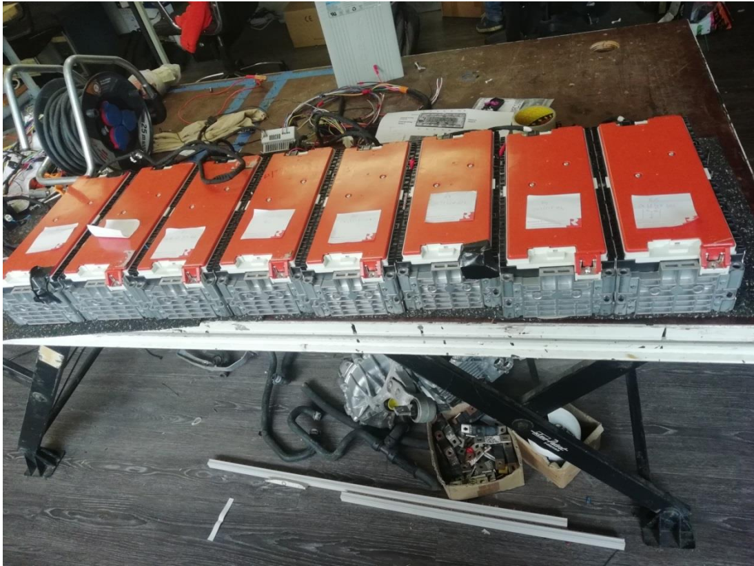
Figure 27 - Series of 8 batteries (different IDs)
