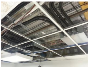
(a) Sensors in ceiling
