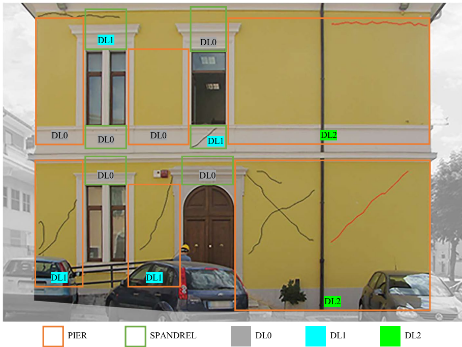
Fig. 2 Assignment of damage levels to structural elements based on the observation of actual damage exhibited by masonry panels, exemplified for a perimeter wall of the Pizzoli town hall building as surveyed after the Central Italy earthquake sequence of 2016–2017 (Sect. 4.3). Black lines represent superficial cracks whereas red lines highlight through-cracks. The average damage level of the wall can be evaluated based on the gravity and extension of damage observed at the structural element scale (Sect. 3.3)
