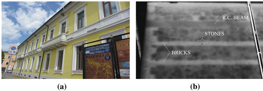
Fig. 4 The Pizzoli town hall building. a View of the façade, highlighting the elongated shape and the regular arrangements of openings on the perimeter walls. b Infrared thermography of a lateral perimeter wall, revealing the masonry typology made up of simple stones with brick courses. A reinforced concrete edge beam is visible at the floor diaphragm level
