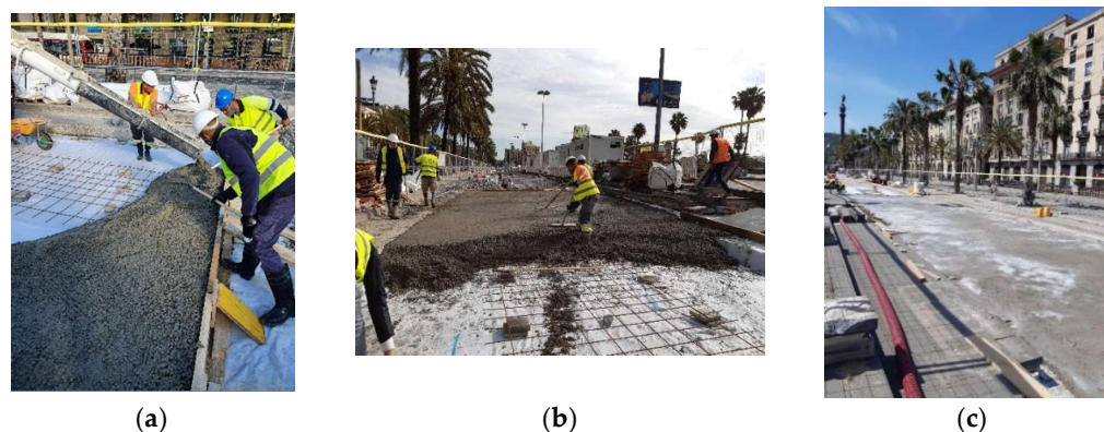
Figure 6. On-site concrete laying (a), compaction (b) and curing process (c) of the concrete.
