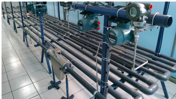
Fig. 8 Experimental pipeline in ITTG (Mexico)
