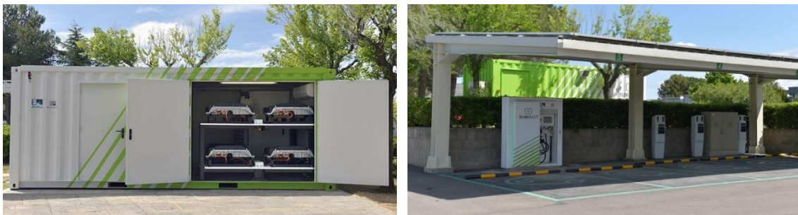
Figure 1. SUNBATT facility in SEAT Martorell. The inside of the SUNBATT container (left). EV chargers (right).
