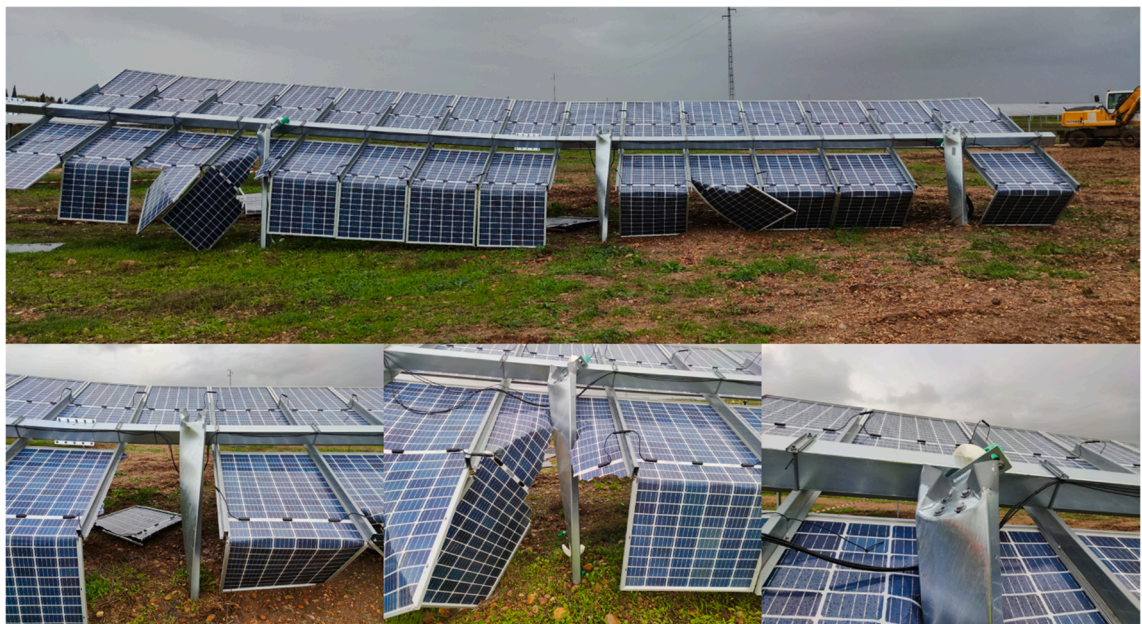
Fig. 6. Detail of the bended and broken PV modules.
