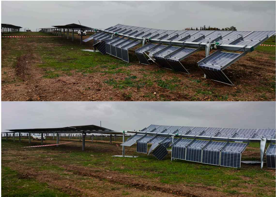
Fig. 3. Damaged solar tracker.
