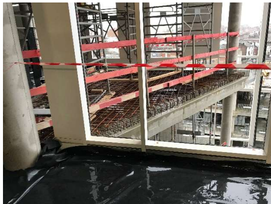
1. A barrier missing on one of the stories of the building.
