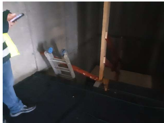
2. An unsafe opening on the staircase shaft.
