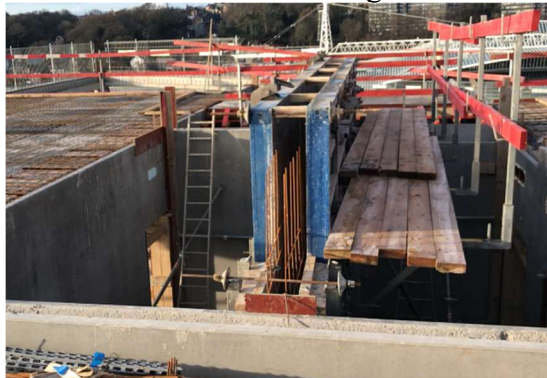
3. Barriers missing on the central core of the building.
