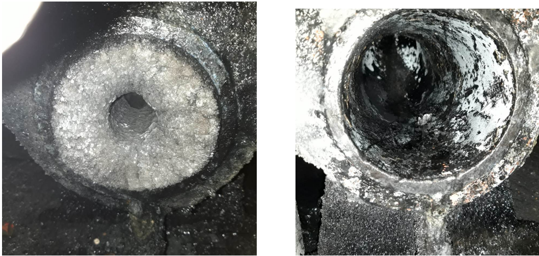
Figure 4.5 Pipelines in AMN WWTP before (left) and after a cleaning stage (right) (pictures provided by AMN WWTP)
