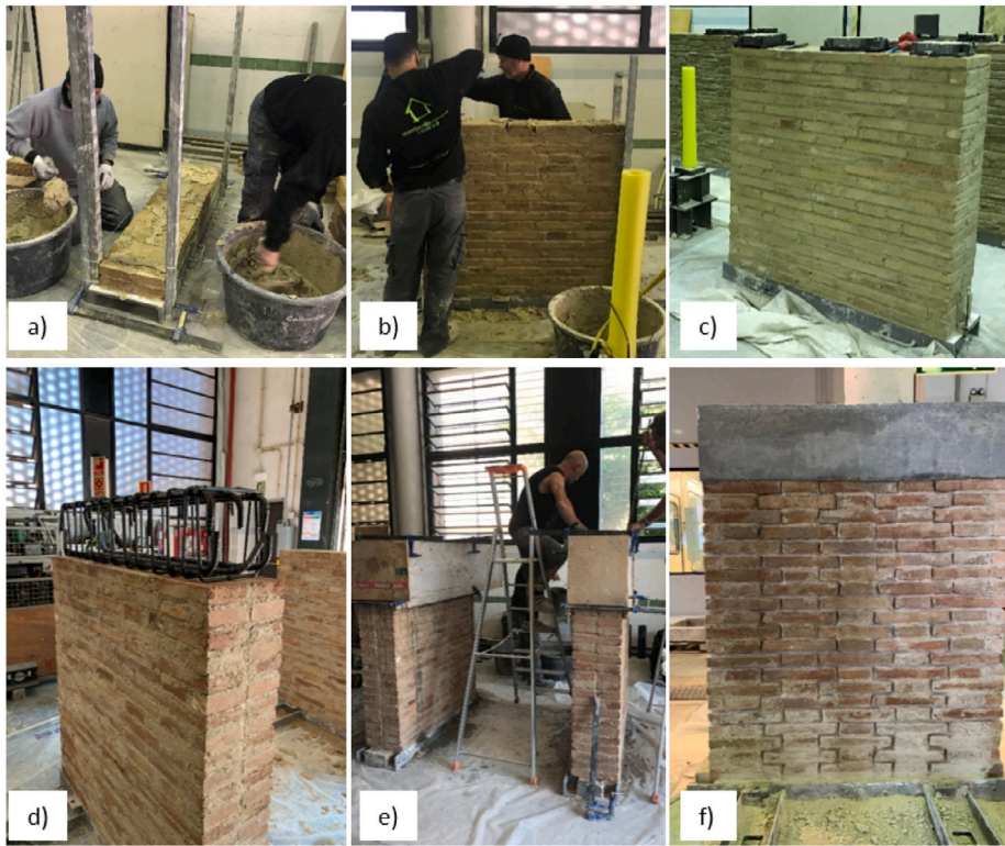
Fig. 1. Construction procedure: (a) placing of the rulers for the construction, (b–c) construction of the wall in Flemish bond, (d) rebars placing for the concrete beam located on top of the specimen, (e) cast of the concrete beam, (f) specimen finished and stored under laboratory conditions.
