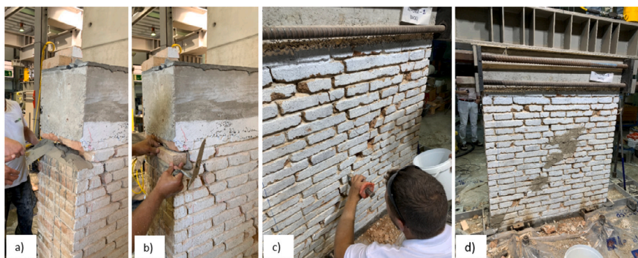
Fig. 3. Scuci-cuci intervention: (a) Removing of fractured units, (b) replacing of fractured units, (c) cracks opening with a hand tool, (d) filling of cracks with lime based strengthening mortar.
