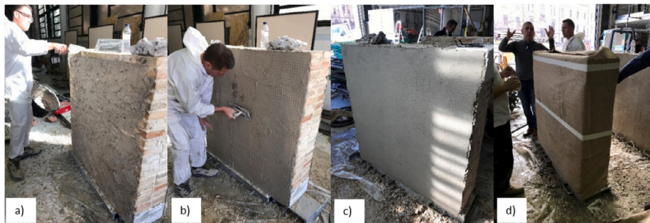
Fig. 2. Procedure for the application of the B-TRM strengthening system: (a) application of the first layer of mortar, (b) set of the basalt grid, (c) finished look of the wall retrofitted with B-TRM, (d) wrapping of the specimens with wet sackcloth fabric for curing.
