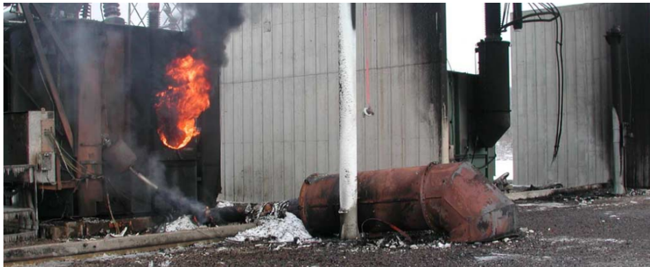
Figure 1.2: Projected chimney due to an internal fault. A chimney in its normal configuration can be seen on the right in the background. Extracted from [12].
