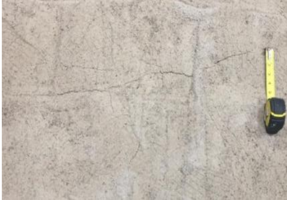
Figure 3.14: Soil failure for 60-mm diameter pipe (1500 mm long specimen: Test D-6)
