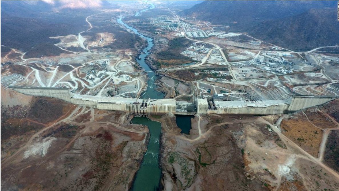
Figure 2: Construction of Grand Renaissance Dam 2017 (CNN 2018. Is Ethiopia Taking Control of the Nile? )
