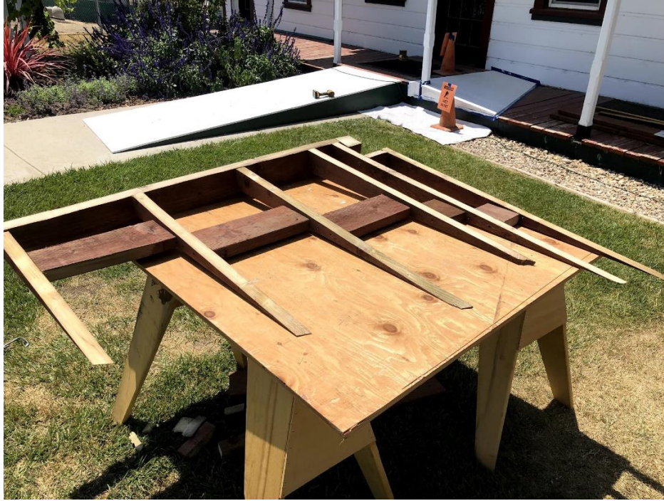
Figure 10: The Framing for One Side Ramp with a Completed Side ramp in the Background
