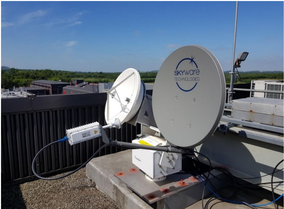
Figure 3-6: Mounted antennas on the Earl Mountbatten roof
