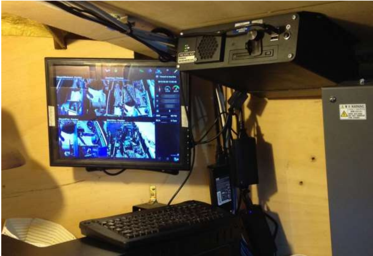
Figure 1.4 A v5 electronic monitoring system installed on a small vessel (photo courtesy of Archipelago Marine Research Ltd.)
