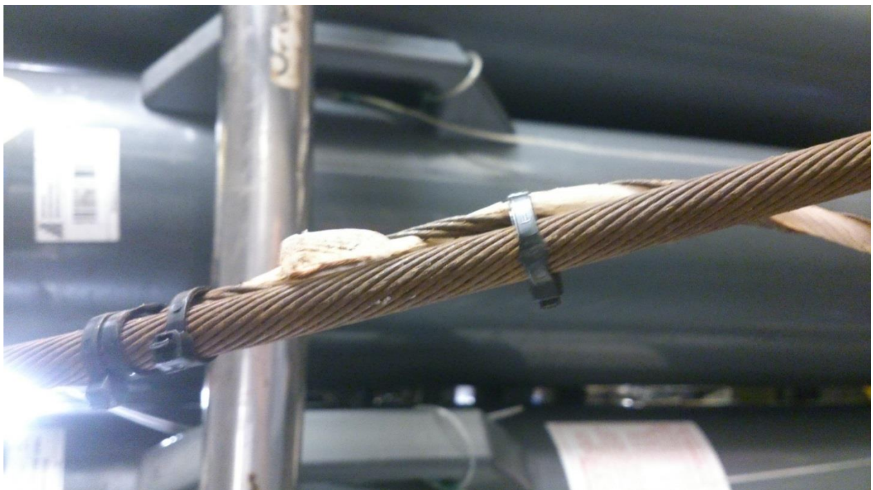
Picture showing the damage caused to the termination when trapped in the roller.
