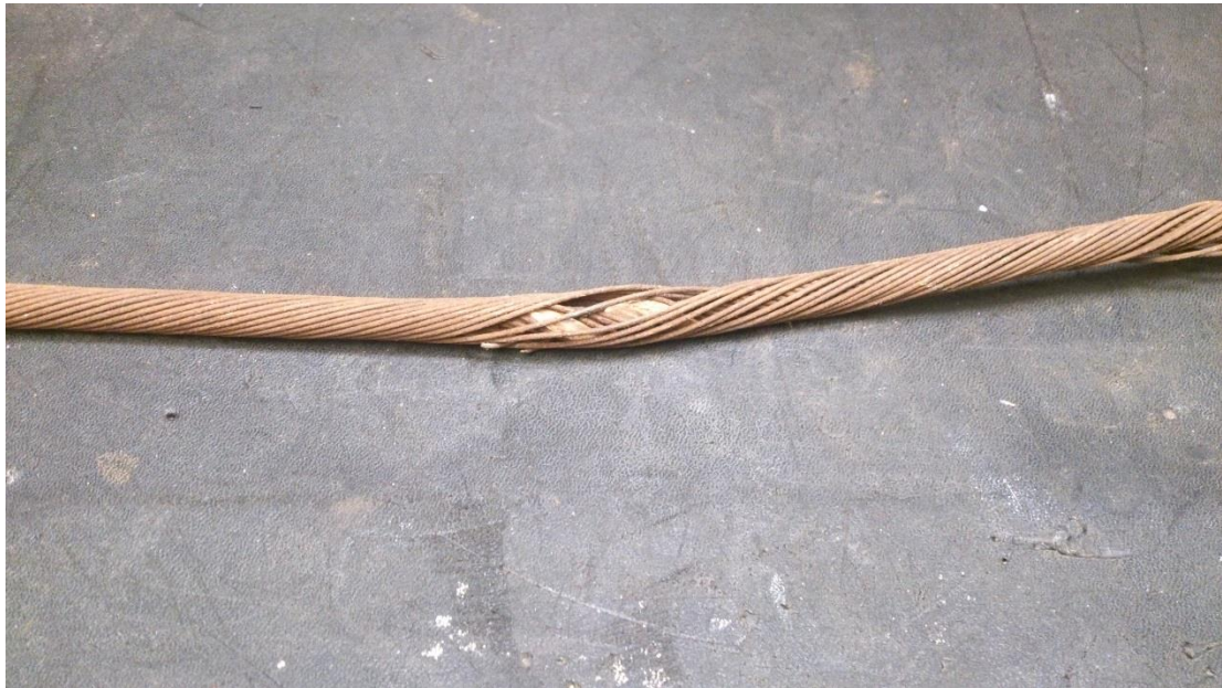
Picture showing the damage to the sea cable at 319m
