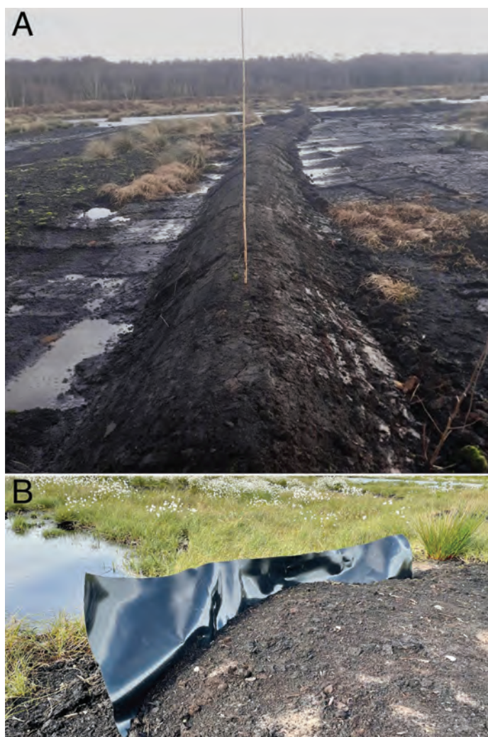
Figure 2: (A) A newly constructed bund, with shallow pools in adjacent scrapes. Credit is due to the skilled and painstaking work of the contractors, not least in employing heavy machinery on a treacherously soft surface; (B) Ply-gene installed in an old ditch line at a bund crossing point; pooled water visible uphill of the ditch block. (Images; M. Longden, A. Osborne).
