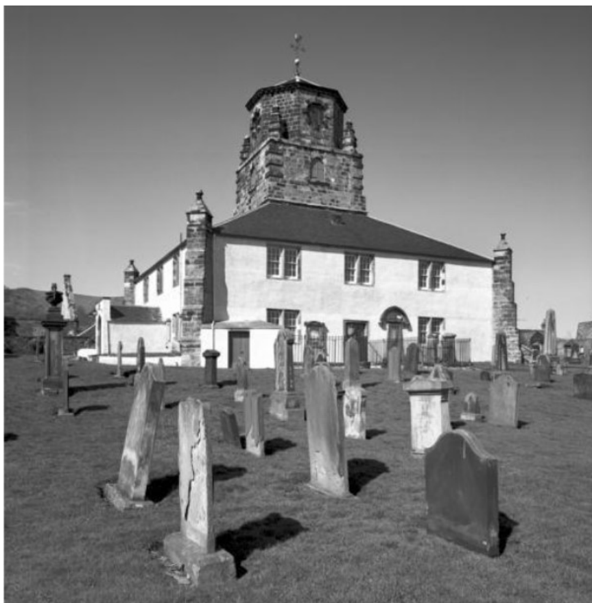
Figure 4.39. The 17 th Century Burntisland Parish Church, with its angled buttresses and octagonal tower.
