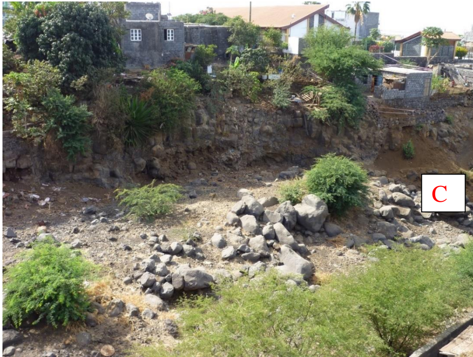
Figure 5.20 A, B and C: Field photos of the western part of Ribeira Domingo Santo (Fogo), showing settlements situated laterally on the edge of channel's left bank. The buildings are on an unstable slope made of layers of boulders (0.5-1 m) which are being eroded and deposited into the channel bed. Direction of the channel and buildings is north to south of Ribeira Santo Domingo (Cape Verde, Fogo).
