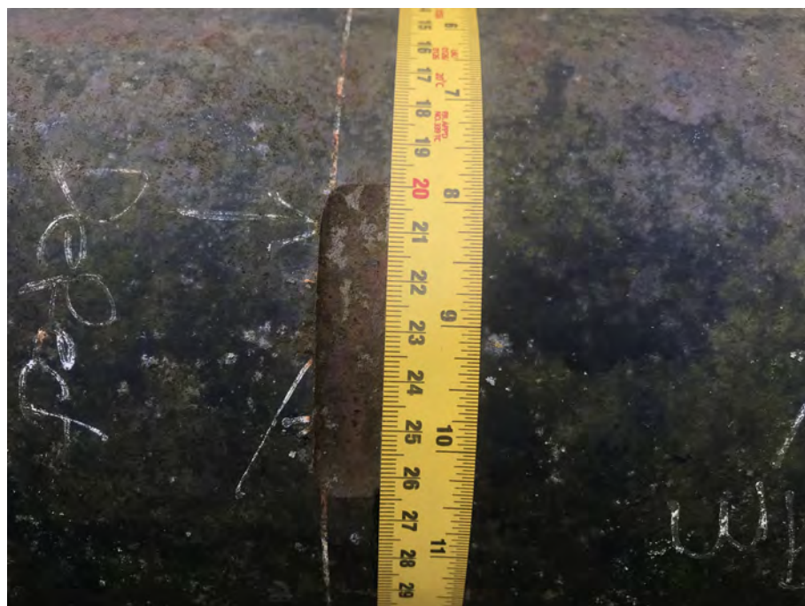
Figure 4.59: The actual appearance of the defect.
