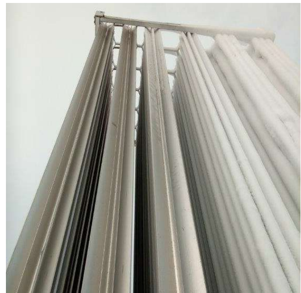
Fig. 1. Longitudinal finned tubes with accumulated ice.
