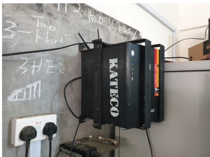
Figure 1. An iBox in situ in a Senior High School in Accra, Ghana.
