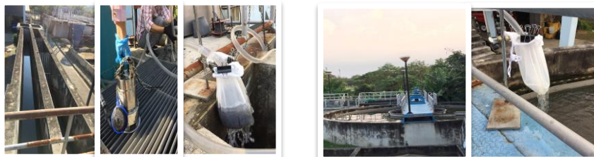
Influent sampling from outlet of automatic fine screen
