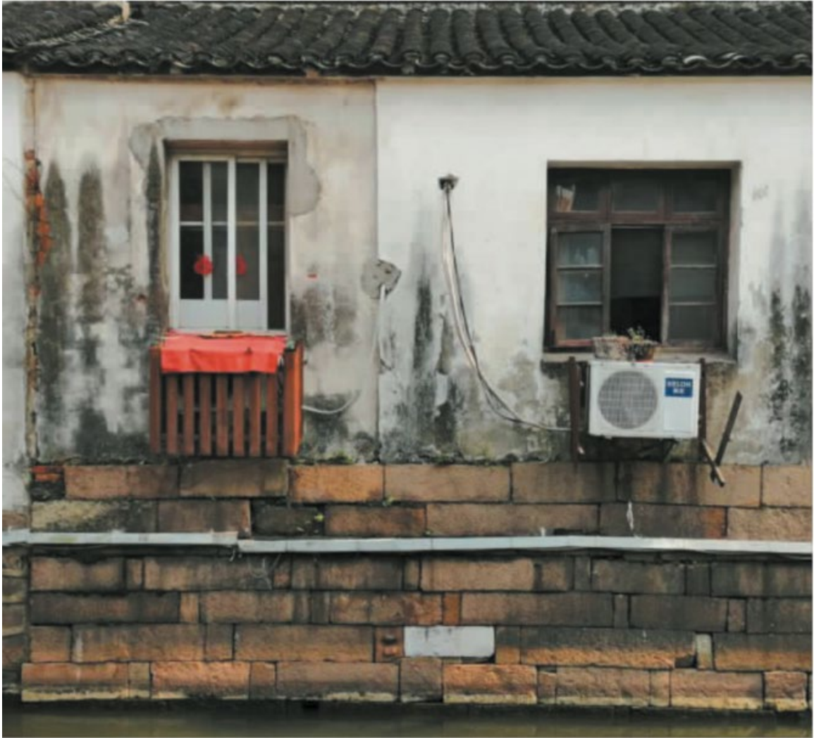
Figure 24-2: Wires, air conditioners, and glass windows on the wall (WU Rongliang. "Analysis of the Problems in the Transformation of Suzhou Shantang Street Historic District [J]." Beauty and Times , 2019(05):37-38.)
