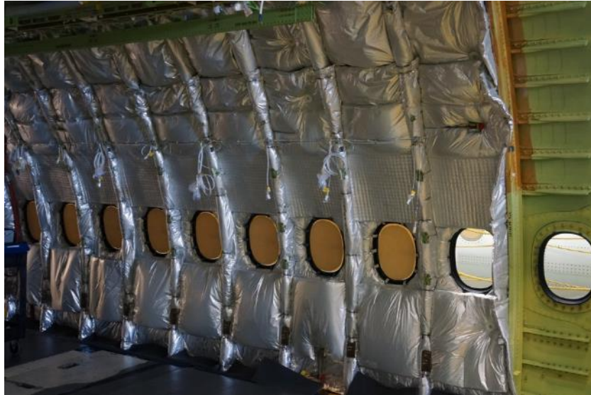
Figure 10 – prefabricated insulation blankets on a Boeing 777 [6]
