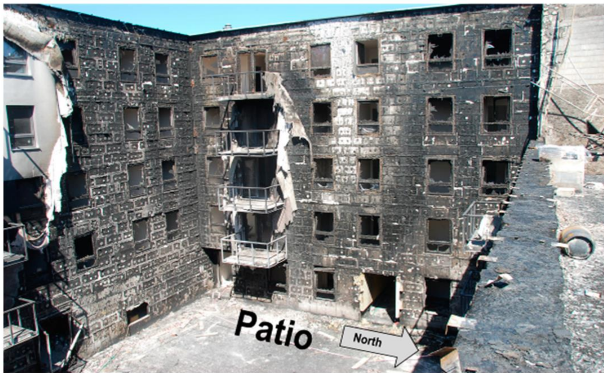
Figure 3.8: Face of 64-apartment complex building after exposure to fire (Wroblewski & Stawiski, 2020)
