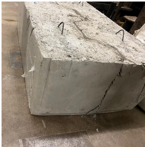
Figure 4. 7:Cracked Concrete Base
