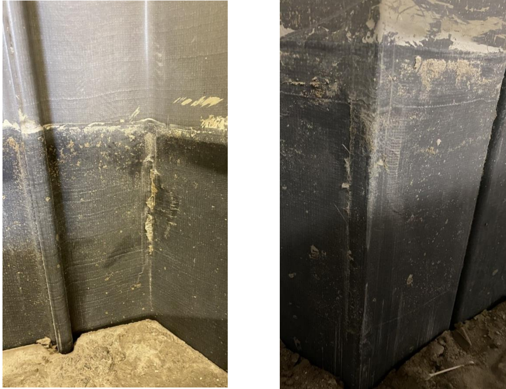
Figure 4. 36:Longitudinal Failures due to Stress Concentrations
