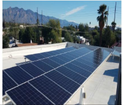
Figure 1. Solar Commons panels on the roof of the Dunbar Pavilion Community Center. (Photo by K. Milun)
