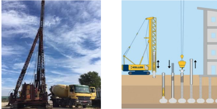
Slika 4. Tehnološki postupak izgradnje FRANKY bušenih šipova Figure 4. Technological process of construction of FRANKY drilled piles
