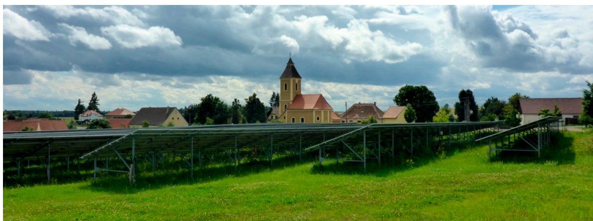
Figure 2. PV plant on the site of a former cowshed. Image by Tomáš Krejčí (Chvalatice, the Czech Republic, 15 May 2021).
