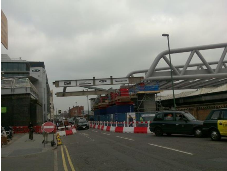
Figure 6-3: NET2 linking to NET1 adjacent to the Nottinghamshire City Hall having been 'slid' over the station.
