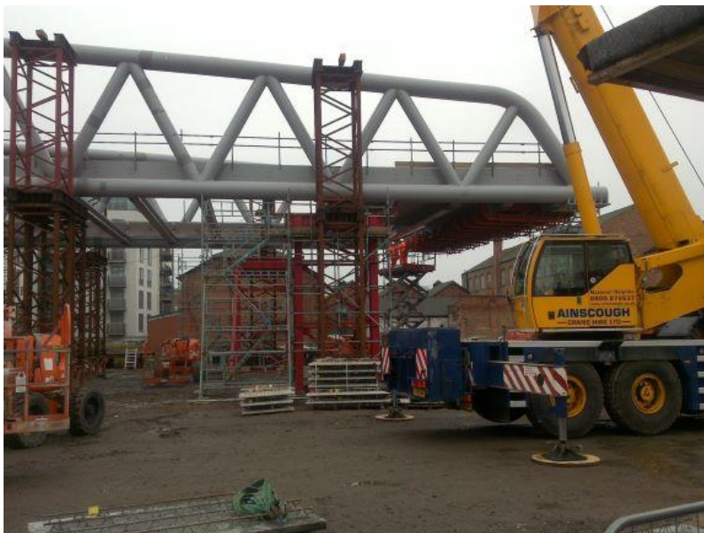
Figure 6-4: Off site construction and assembly of the tram overbridge adjacent to Nottingham Station
