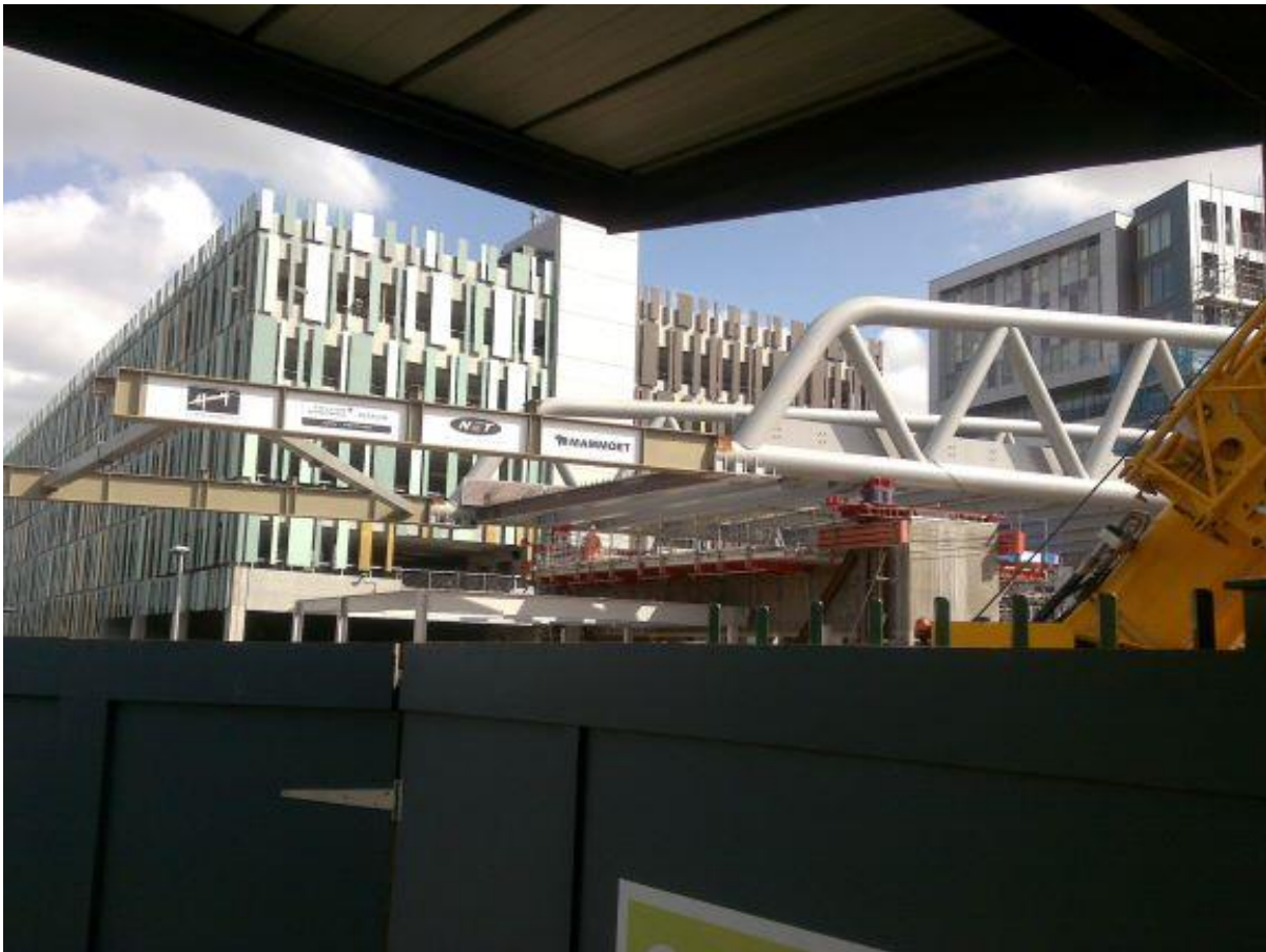
Figure 5-8: Car Park in background with NET2 overbrige in foreground during the process of installation over the station
