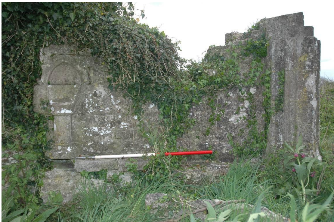
Figure 4: Interior east wall of the south porch showing the relative locations of the stoup (left) and the stone bench. The dip in wall above indicates the former position of the quatrefoil window. Ivy ( Hedera helix ) is firmly rooted into the top of the fabric.
