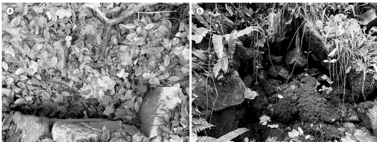
Slika 7a i 7b. Urušeni 'drugi tip' vodopropusnoga objekta Fig. 7a and 7b Collapsed 'other type' of water-permeable structure
