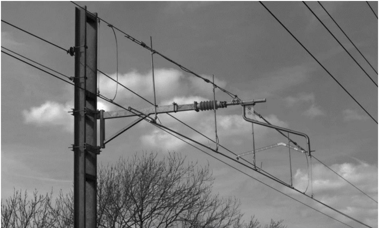
Figure 6.1 Neutral section installed at Old Dalby from DBST trackside video. Note the 'lever arm' at the nearer end.
