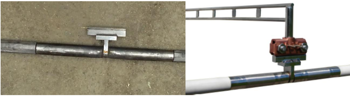
Figure 6.8 Centre connection between CW insulators showing registration arm attachment
