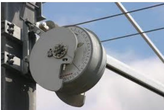
Figure 2.21 Spring tensioner equipment used on Network Rail series 1. (source Pfisterer)
