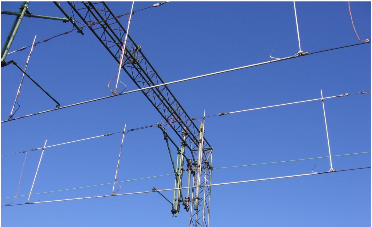
Figure 3.14 Photograph of Arthur Flury single rod neutral sections in adjacent tracks. Note the absence of lever arms. From (Dolphin, 2014)
