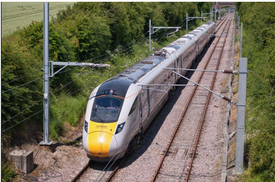
Figure C.1 Hitachi IEP train on test at Old Dalby. Furrer+Frey Series 1 OCL installed on Up (northbound) track, on LH side in the photo (Photo credit Barry Duffin)
