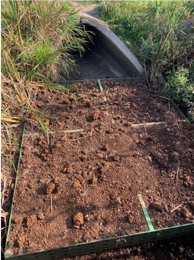
Figure 5. Pilot scale steel byproduct filter May 2020.
