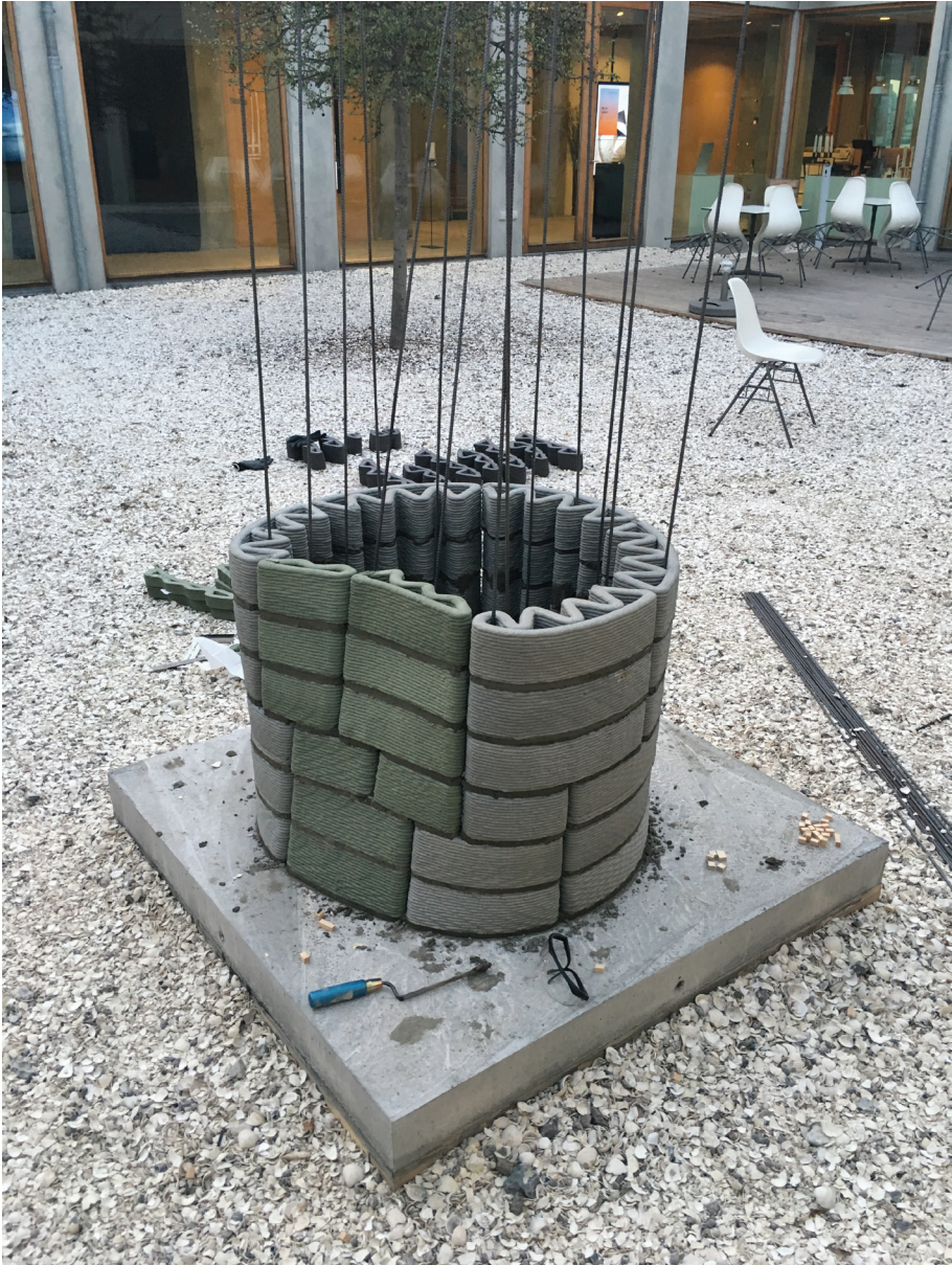
Figure 4.5. The full-scale concrete demonstrator during assembly. Vertical steel rods anchored in the concrete base are added to the construction to ensure structural integrity. Photo by Mads Brath Jensen.
