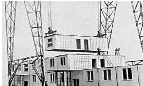
Fig.4 – Mounting volumetric blocks. Source: Ataev. 1967. Technology and Economics of Volume-Block House Construction
