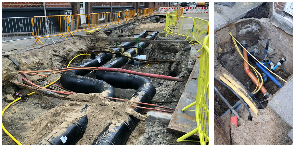
Figure 5: Big utility lines are often not explicitly described on 2D line representations on utility maps, and can sometimes be located closer to the surface than expected.
