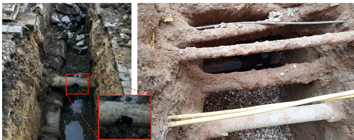
Figure 6: Damage on old utility line on the left and corrosion on utility pipes on the right.
