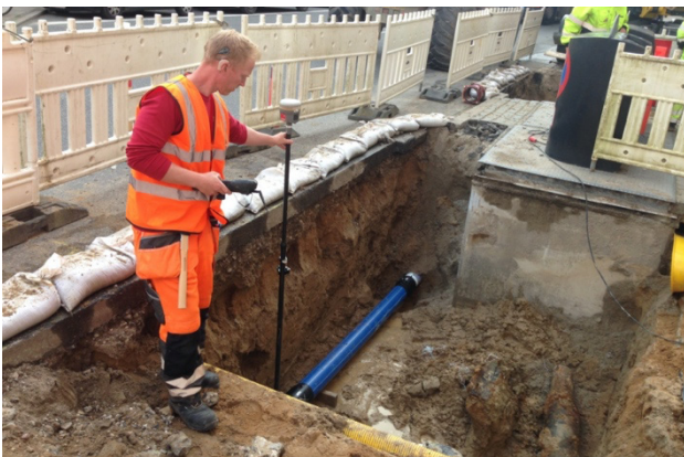
Figure 1. Surveyor using conventional GNSS-RTK equipment to survey a newly placed water pipe.
