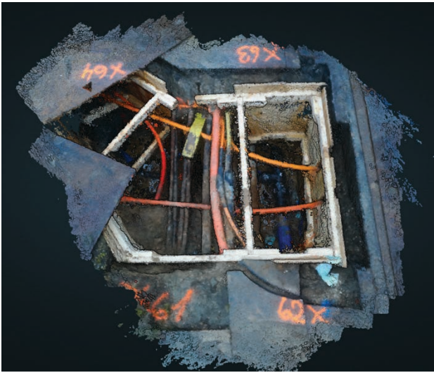
Figure 7. Point cloud capture of an excavation hole containing as-built water pipes (blue pipe in bottom) with other types of utilities crossing over.
